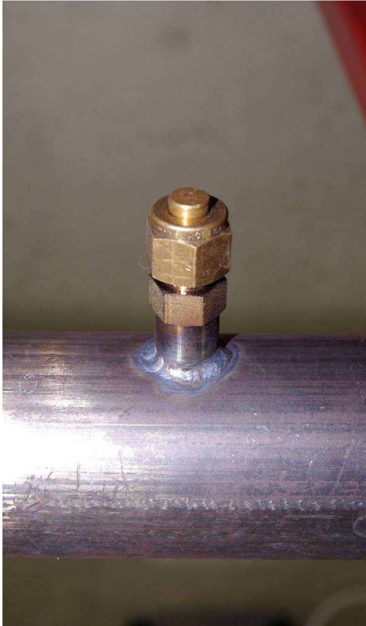
Figure 2 Swagelok fitting welded into exhaust, with blanking plug fitted
